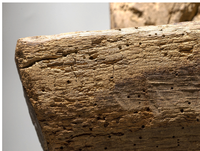
Fig. 2. The underside of one of the cross-braces, which is worn and shows traces of fungal and wood worm attack (Photo: Rijksmuseum).
